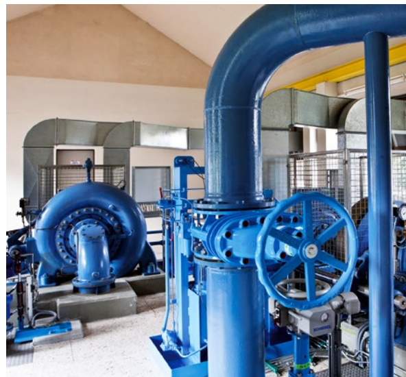
Hinternasswald power station
